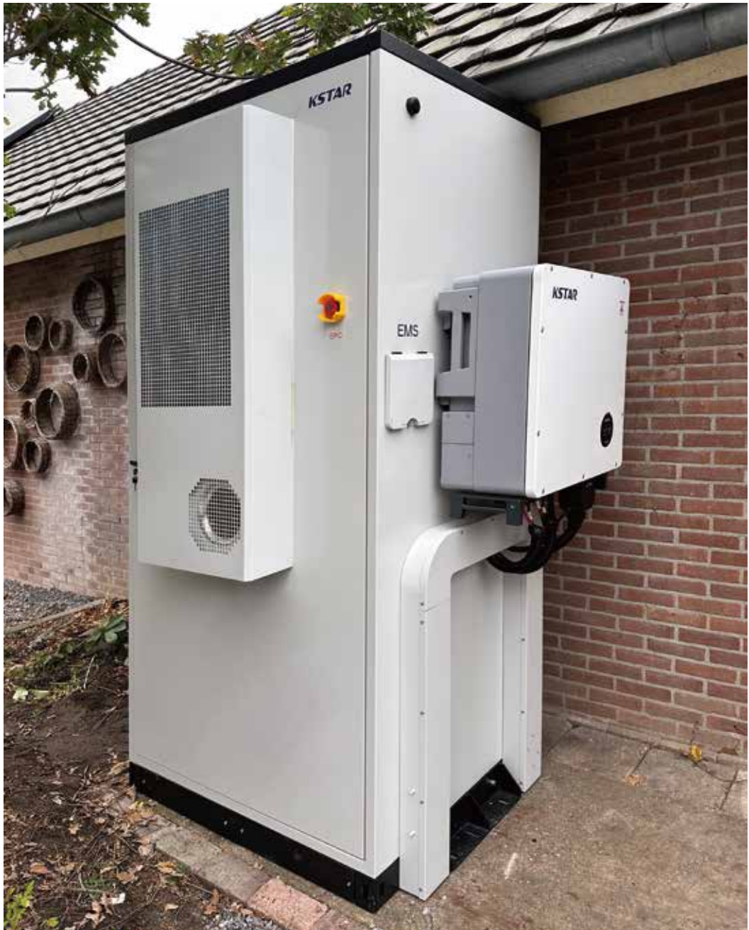
08 C&I ESS Project in the Netherlands
