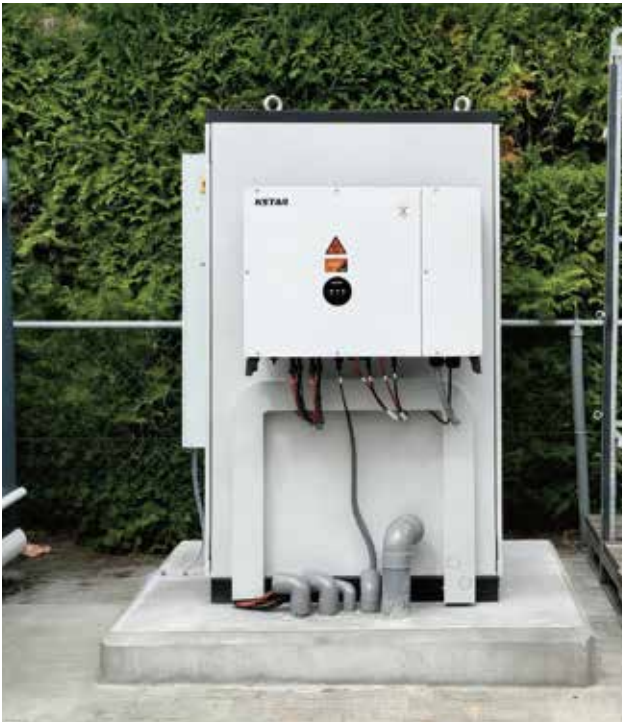
01 C&I ESS Project in the Netherlands
