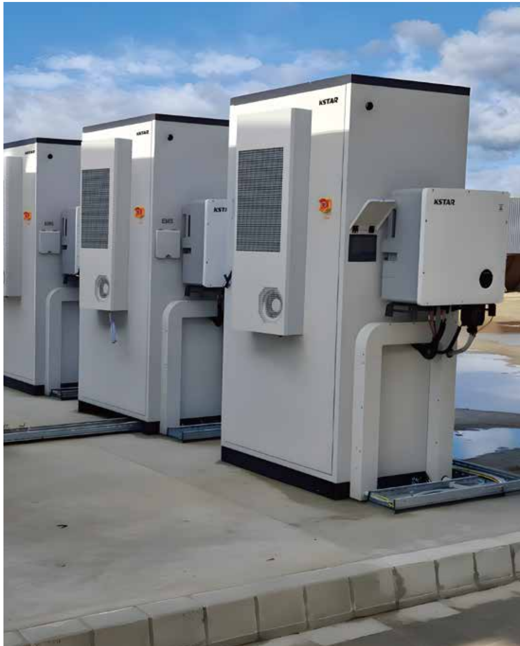
07 C&I ESS Project in Hungary
