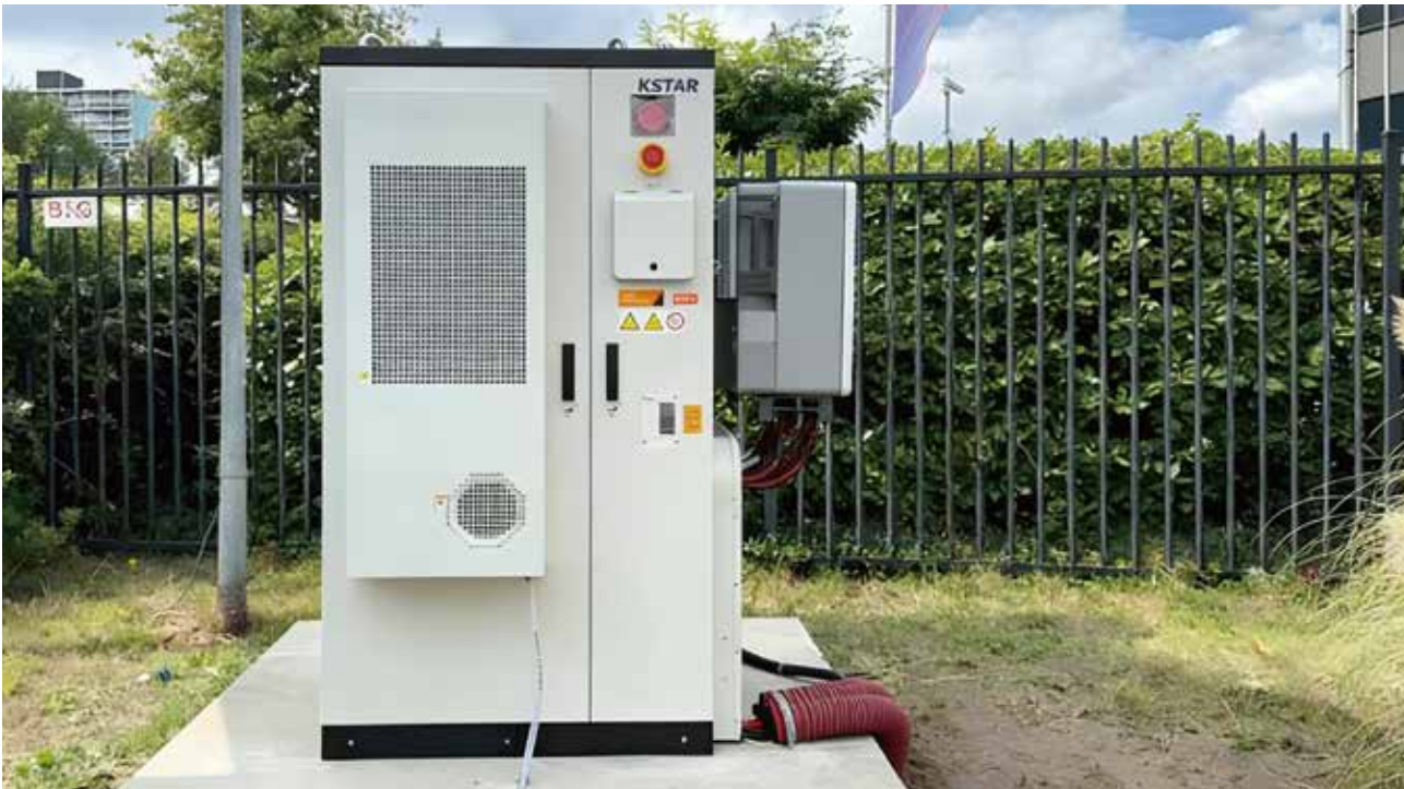
04 C&I ESS Project in the Netherlands
