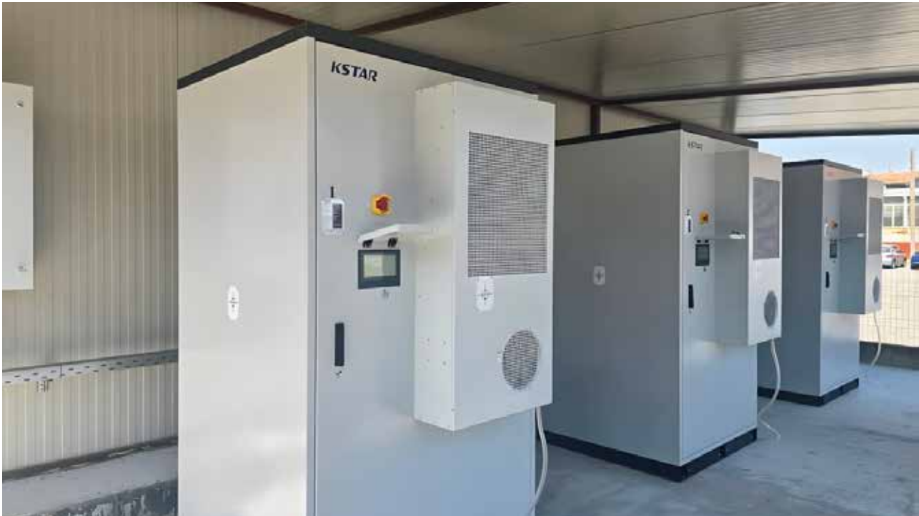
03 C&I ESS Project in Bulgaria
