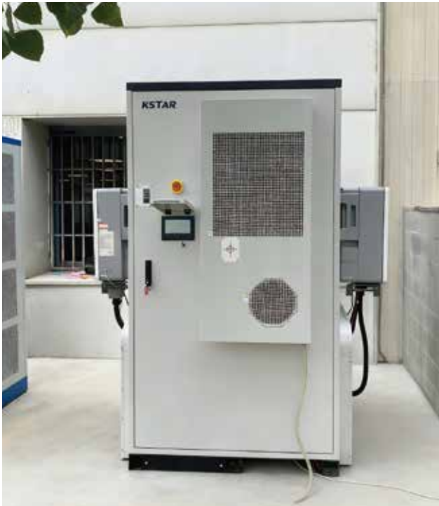
02 C&I ESS Project in Spain
